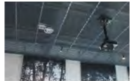
Air-conditioning and ventilation
